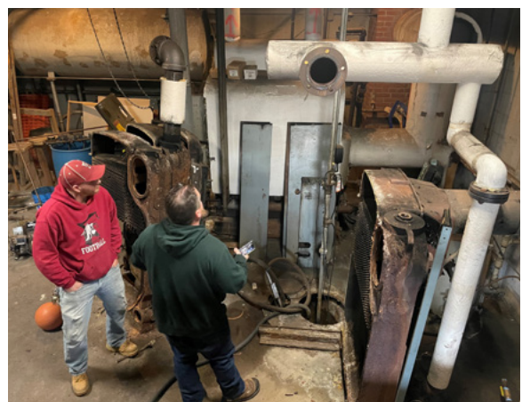
Old HVAC systems like the one shown here are common in municipal buildings that were used in the mid-20th century. These systems often require oil tank and asbestos removal as part of any re-use or demolition.
