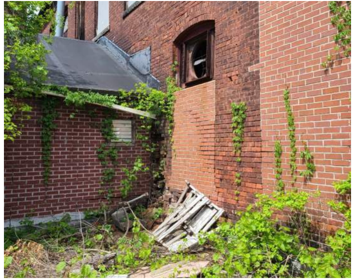
8 Building 7 & 8 Deteriorated Exterior Walls
