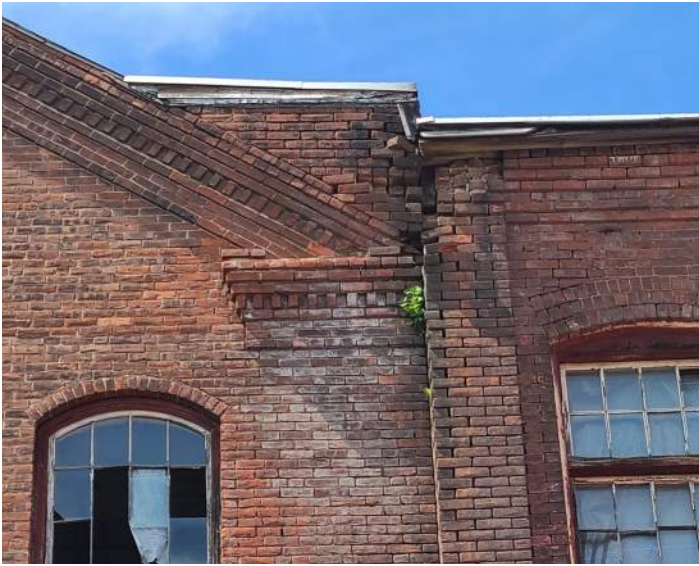
7 Building 5 Exterior Brick Failure
