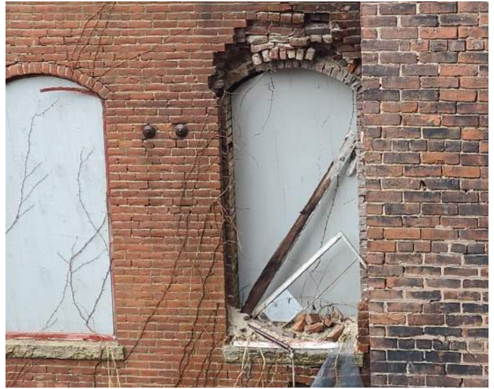
2 Building 1 Failing Window Arches
