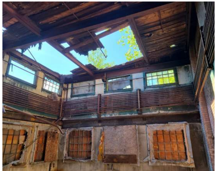
4 Building 11 Addition Collapsed Roof
