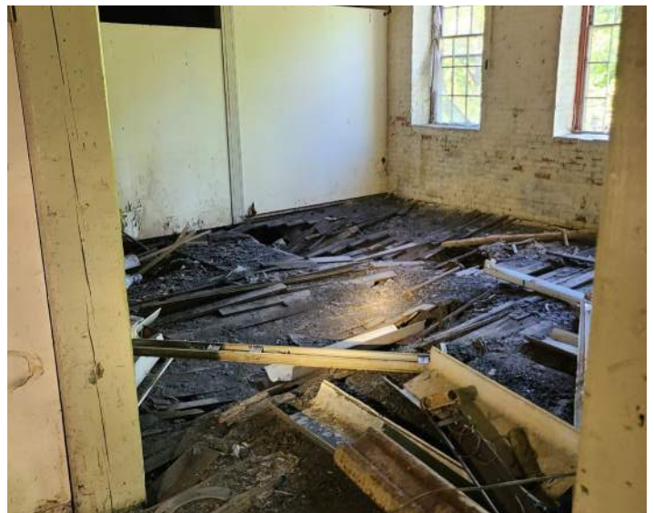
6 Building 1 Collapsed Floor System
