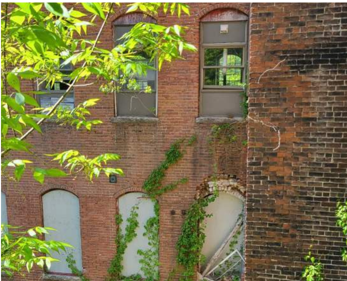
9 Building 1 Failing Window Arches and Elevator Shaft
