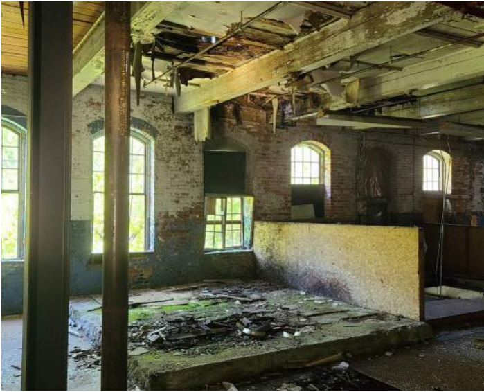
13 Building 2 Collapsed Ceiling
