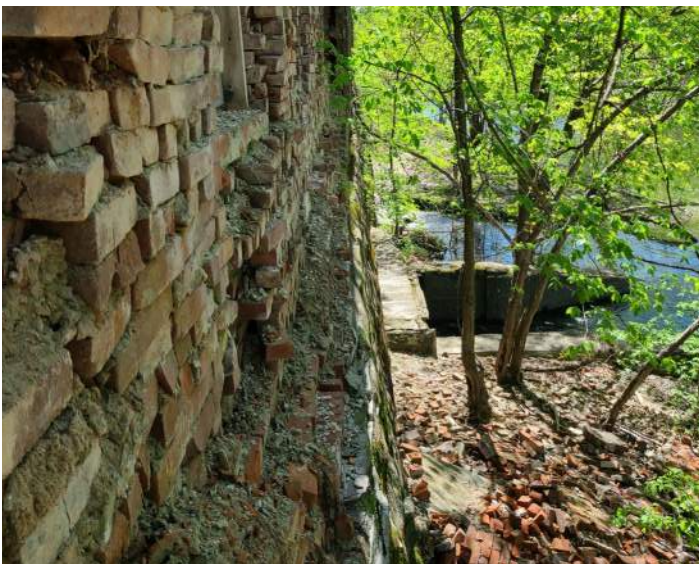
11 Building 2 Deteriorated Exterior Brick Wall System at River-side
