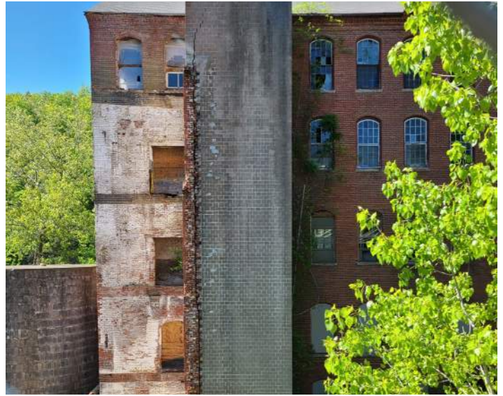
14 Building 1 Wall of Elevator Shaft Separating
