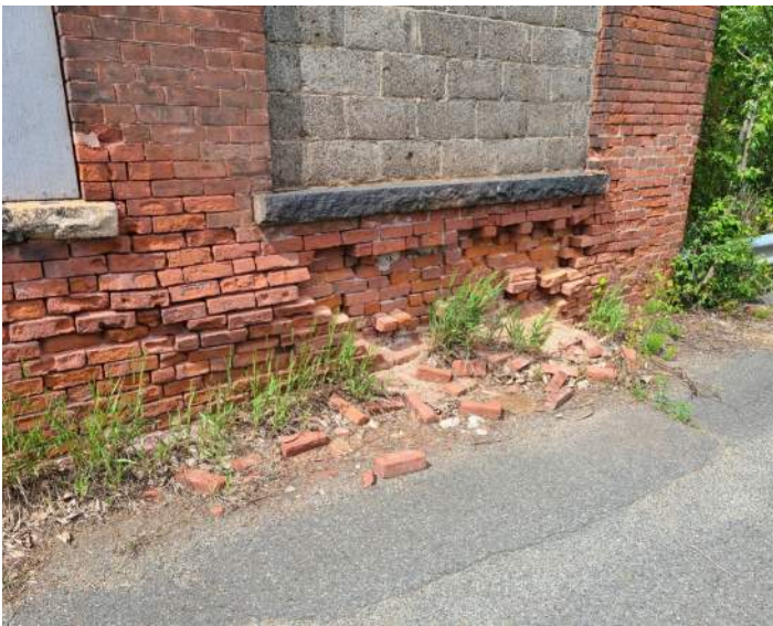
3 Building Exterior Wall's Outer Wythe Falling Out of Base
