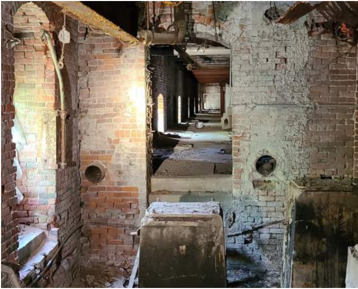
1 Building 3 Deteriorated Brick and Mortar
