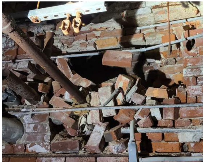
10 Building 6 Crumbling Brick and Utilities
