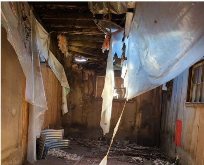
15 Building 11 Failing Ceiling and Deteriorated Interior Finishes
