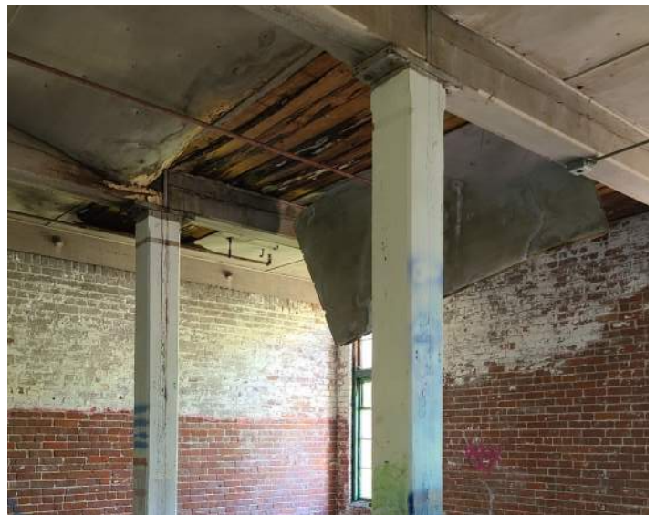
16 Building 11 Floor Assembly Failing at Corners
