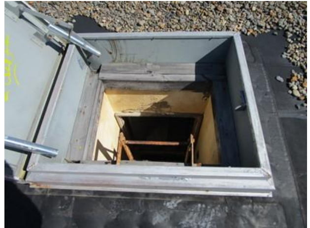
14. Roof hatch has very small opening and offsets at ceiling level.
