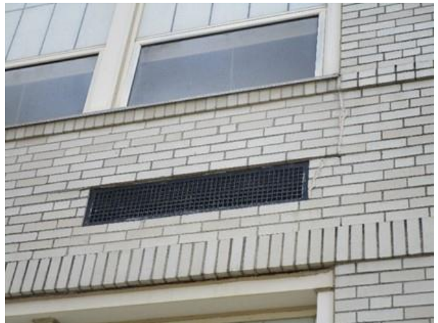
10. Brick cracks and displacement were typically observed at classroom vent openings.
