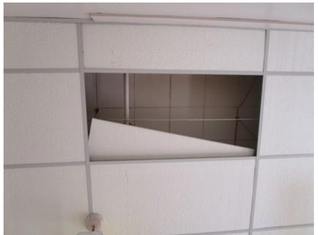
16. Existing ceiling consists of original spline ceiling tiles with new acoustical ceiling grid and tile system installed below.
