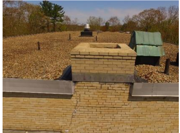
8. Isolated area of cracked and displaced masonry on south wall at chimney above low roof.
