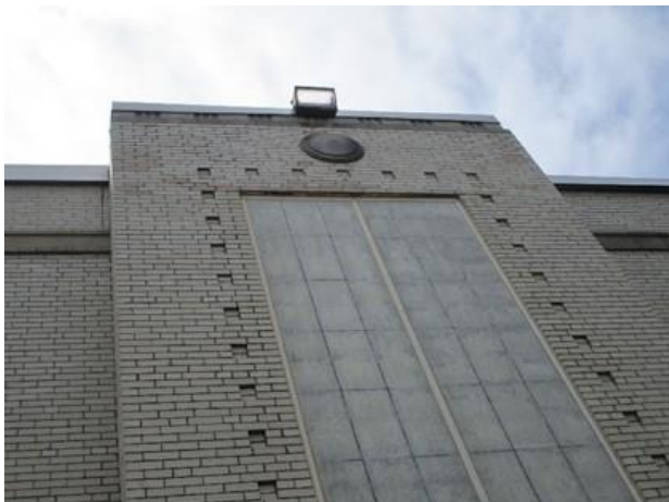
11. The Kalwall windows are in poor condition with extensive fiber bloom on the exterior lamination.
