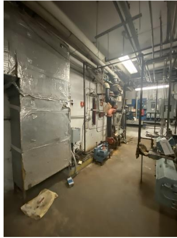
26. Boiler room in basement.
