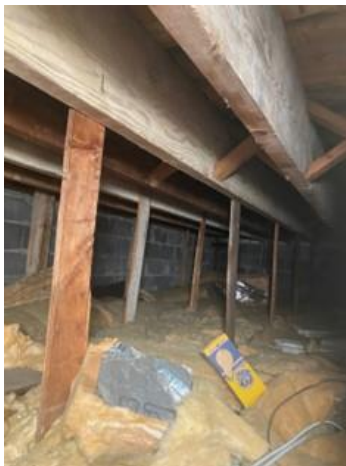
15. View of roof framing near roof hatch, with plywood strips used to hang ceiling joists.
