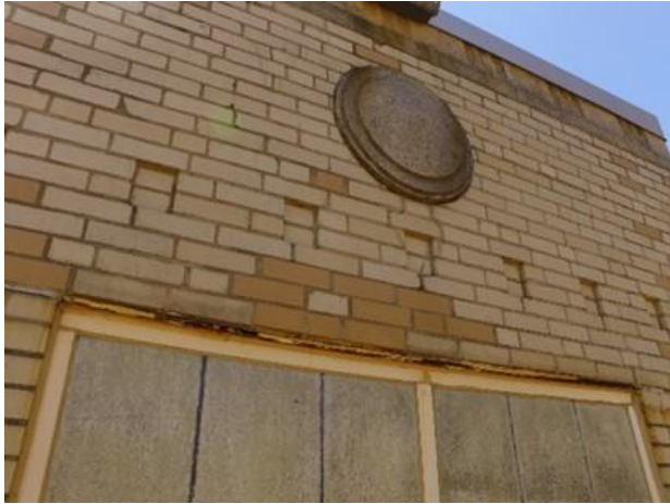
7. Lintels are rusted, with rust formation starting to displace brick masonry.
