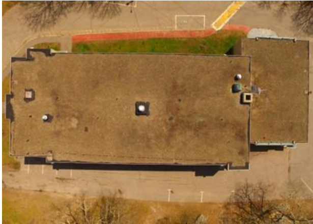
13. Overall view of the roof area, with ballasted EPDM roof membrane at the end of its lifespan.
