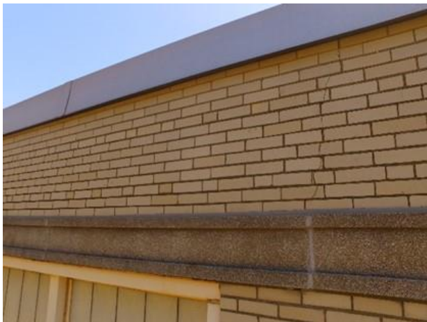
9. The brick façade is generally in good condition, but there are isolated cracks throughout the façade.
