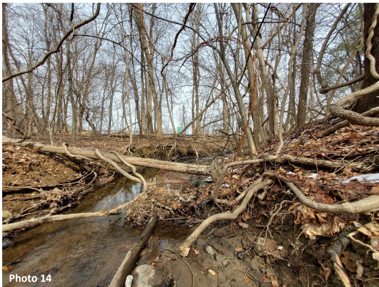
Photo 14 shows the stream channel as it approaches the culvert under Water Street (Photo 12). This is an areas where the banks appear to be less stable and susceptible to erosion.
