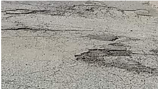
Picture 1: Pavement Deterioration
