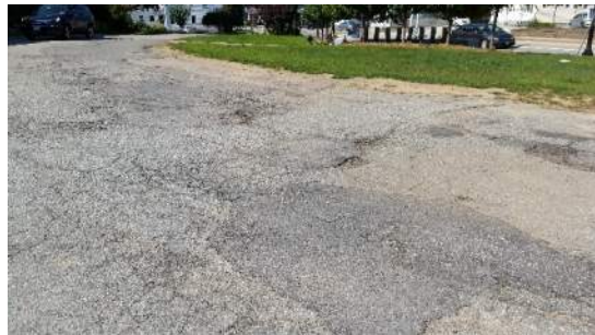
Picture 2: Pavement Deterioration
