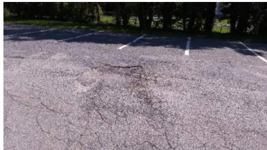
Picture 6: Pavement Deterioration
