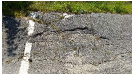
Picture 4: Pavement Deterioration
