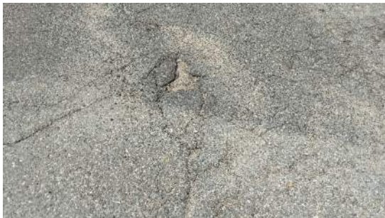
Picture 5: Pavement Deterioration
