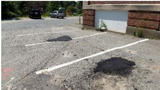
Picture 3: Pavement Deterioration
